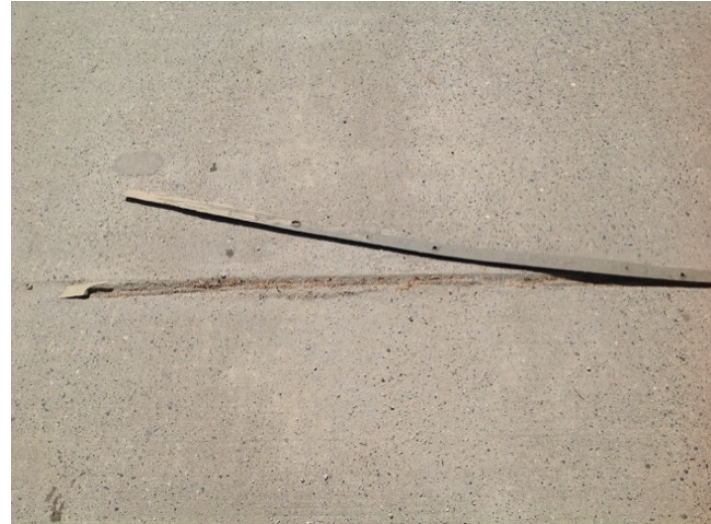
sealant worn and failing
